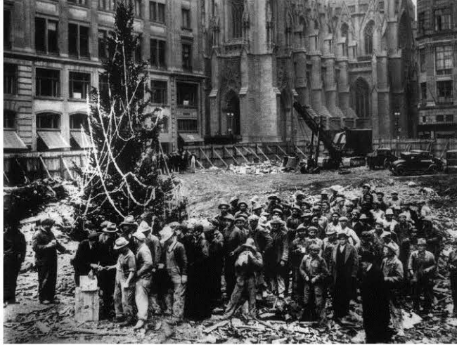
Workers excavating the site for Rockefeller Center in Midtown lined up by a Christmas tree, the first mounted there, on Dec. 24, 1931. Associated Press
